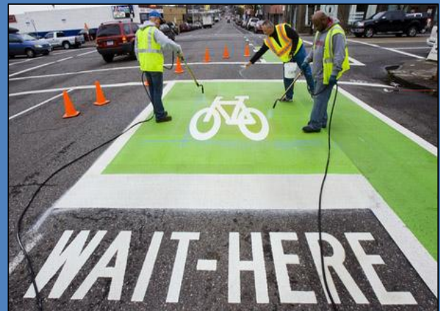
Bike boxes, like the one above being installed in Seattle, are still considered experimental, and require education for both drivers and bicyclists.
