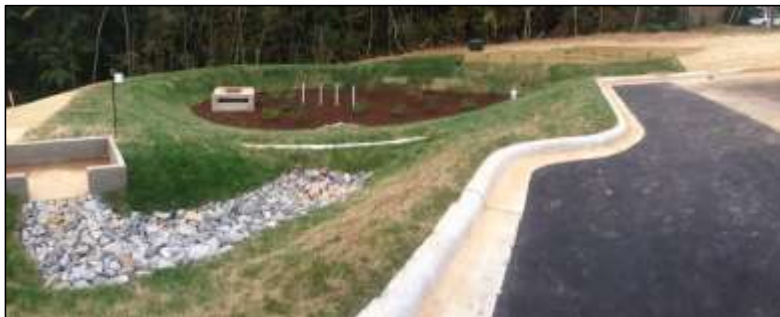
Figure 4.2-3 Bioretention Area Near Parking Lot
