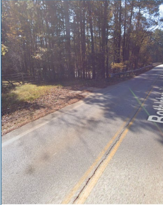
Cracked pavement at possible fire access on Bethlehem Road.
