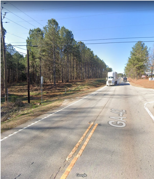
Site entrance pavement conditions on SR-42 on intersection with Pine Grove.
