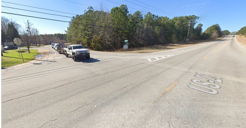
Pavement cracking on intersection of US-23 and Bethlehem Road.
